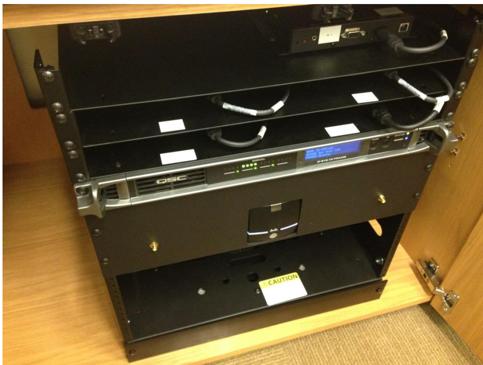
Figure 8: Example of wrong ClickShare installation: the antenna are not connected on the ClickShare rack-mounted kit
