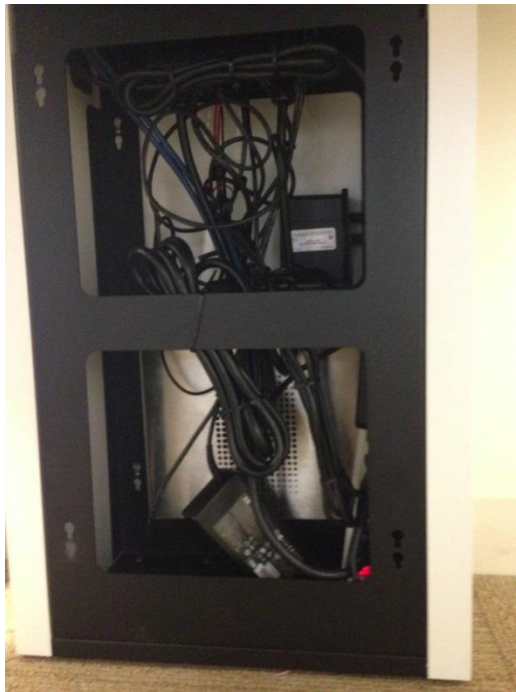
Figure 10: Example of wrong ClickShare installation: the base unit is placed inside a metallic closet without using antenna extension kit which strongly deteriorates the signal quality
