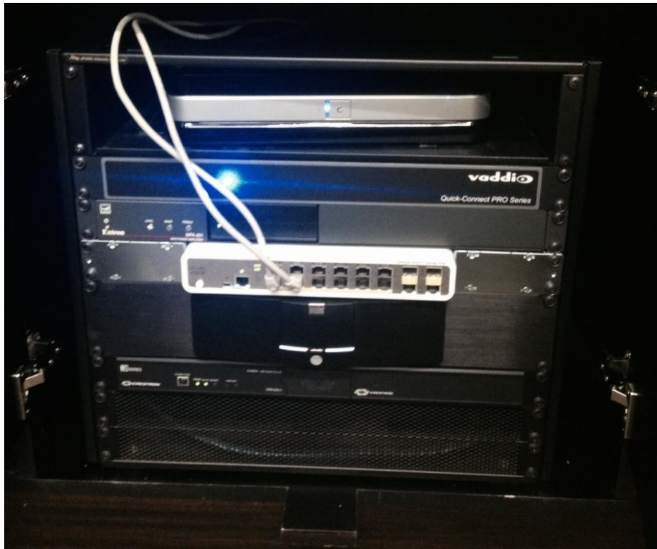
Figure 9: Example of wrong ClickShare installation: an incorrect rack-mounted kit is used and the ClickShare base unit antennas are enclosed in the shelf
